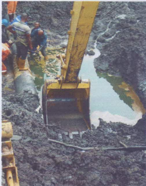
SPILL DURING REPAIR: fig2
